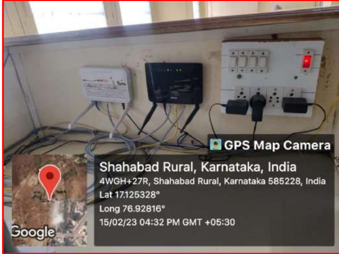
Fiber Optics Internet connection in Office
